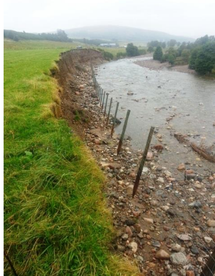
Bank erosion on the River Avon caused by a recent spate.
